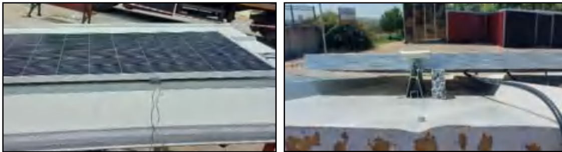
Figure 9. Temperature sensors installed on the PV system
