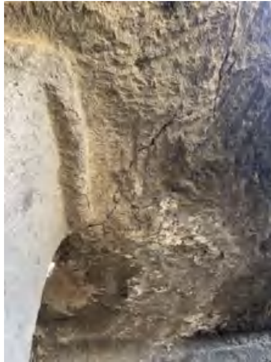
Figure 2. Crack type deteriorations observed in the monument
